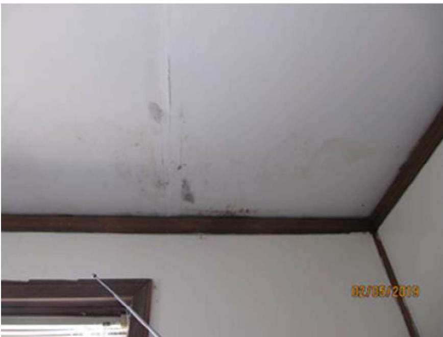
Building Interior Water Damage
