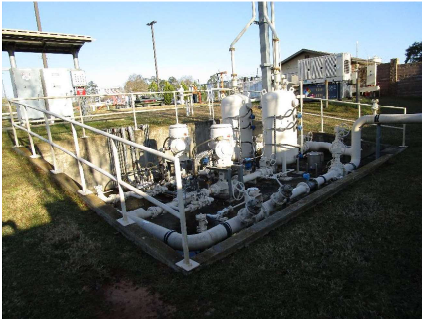
Fill Stand Exposed to Elements
