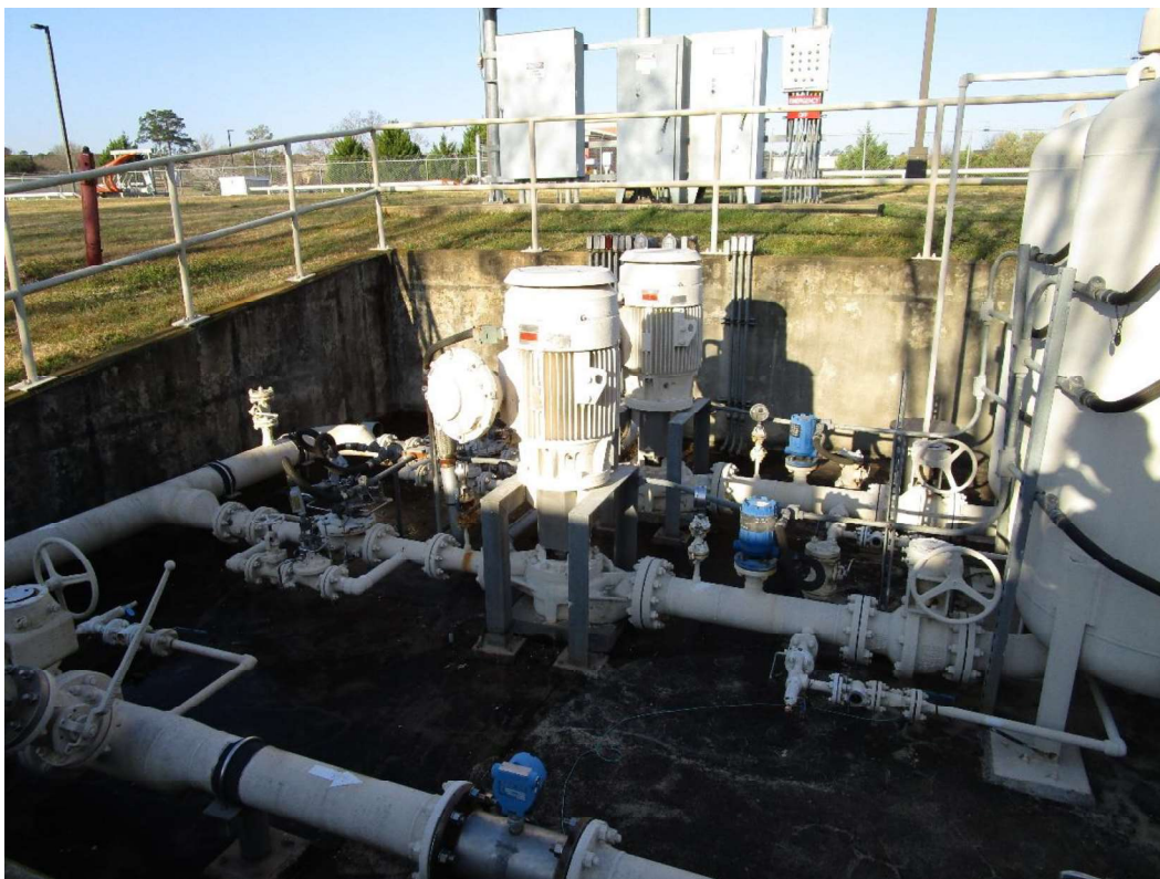
Filter Equipment Pad Exposed to Elements
