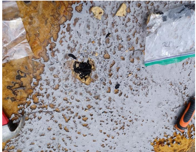
Photo 26: View of the yellow insulation and black roofing on the western roof.
