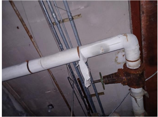
Photo 22: View of the asbestos containing white insulation on the basement piping and showroom pipe elbows.
