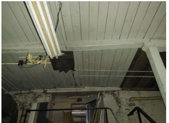
Photo 10 – Typical view of the white wooden ceiling in the area of the basement storing kegs of beer – LBP
