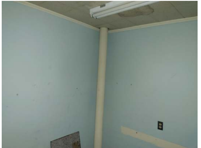
Photo 8 – Typical view of a white metal vertical pipe found in the room with blue walls next to the vault – LBP
