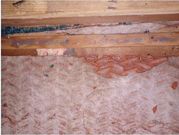
Photo 15: View of the red carpet backing in a portion of the office area.
