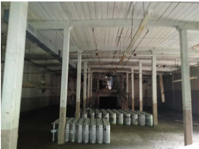
Photo 9 – Typical view of the white wooden ceiling in the area of the basement storing kegs of beer – LBP
