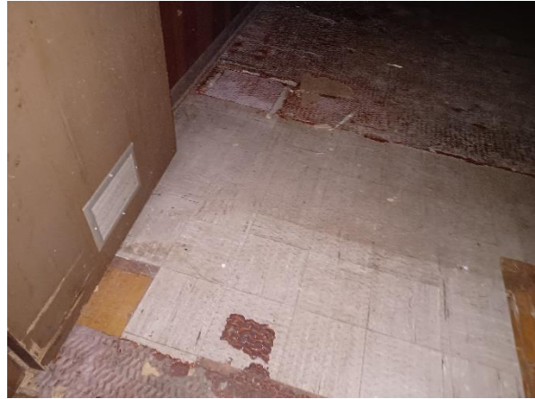
Photo 16: View of the tan floor tile and underlying asbestos containing brown mastic in select office area rooms.
