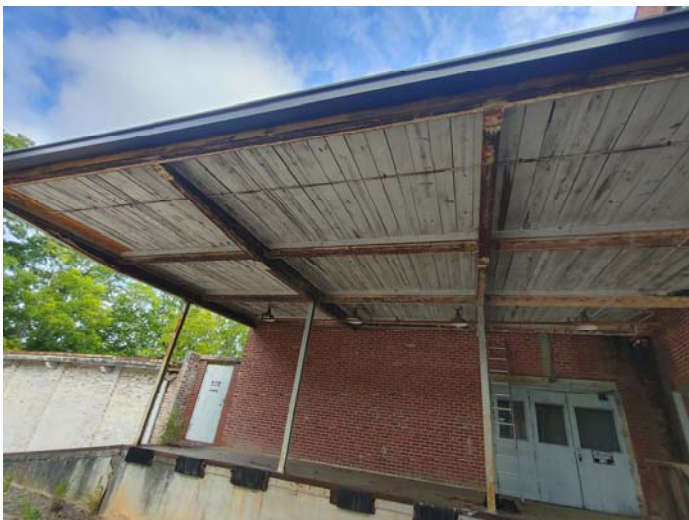
Photo 5 – Gray wooden awning ceiling & gray metal I-Beams at the loading dock – LBP
