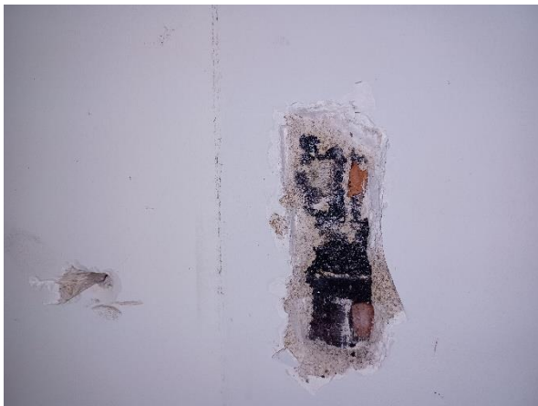
Photo 11: View of the white plaster skim coat, tan plaster base coat, and black tar located along perimeter walls in showroom and portion of office.
