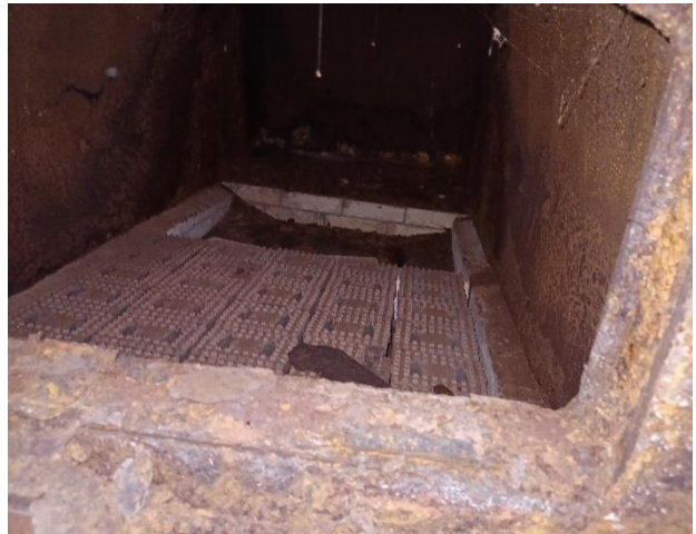
Photo 24: View of the presumed asbestos containing fire brick located within the furnace.
