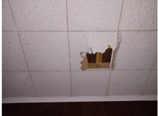
Photo 14: View of the white, tan ceiling tile in the office area.
