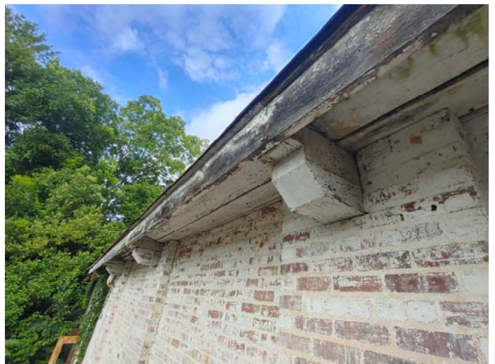
Photo 6 – White brick walls & white wooden corbels, soffit & fascia in the loading dock area – LBP
