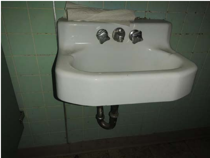
Photo 7 – Typical view of a white metal sink found in the bathrooms – LBP
