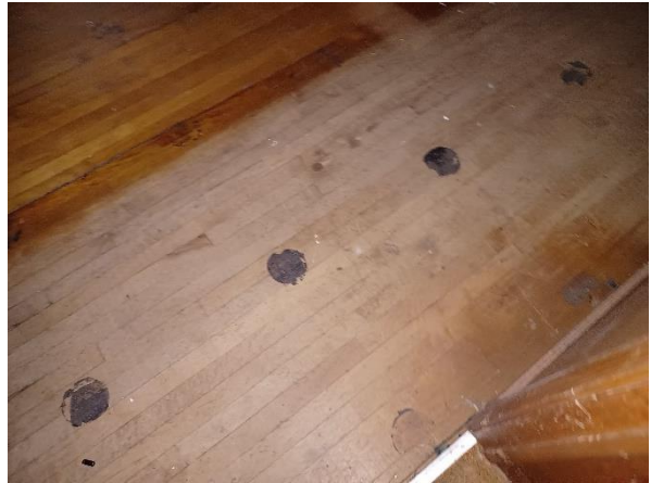
Photo 18: View of the black mastic pucks in one room in the office area.
