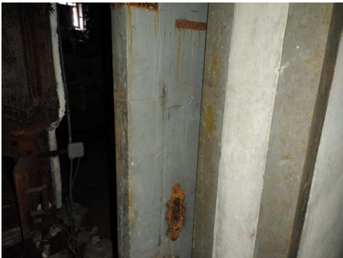
Photo 11 – Typical view of the gray metal fire door in the boiler room within the basement – LBP
