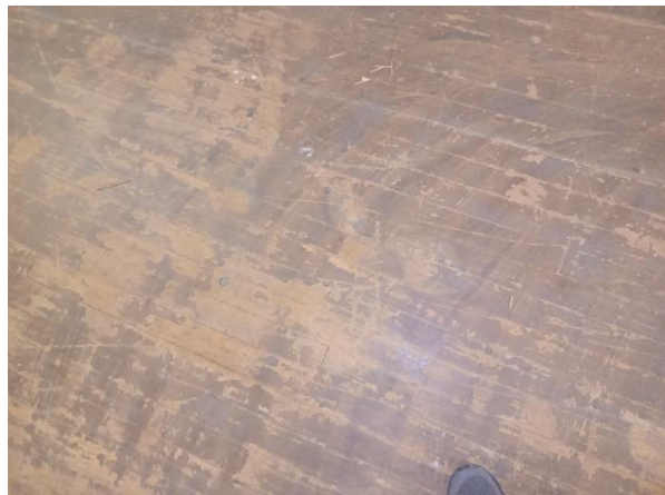
Photo 12: View of the brown mastic in the showroom.
