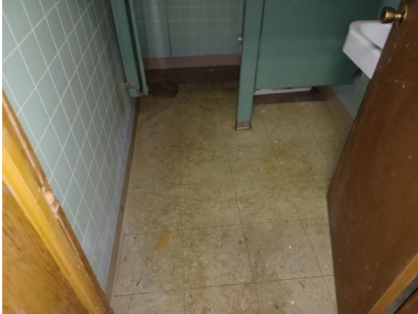
Photo 13: View of the asbestos containing white floor tile and underlying black mastic in the showroom bathrooms.
