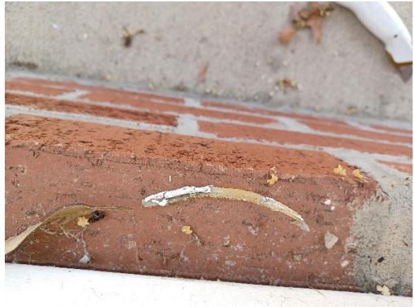
Photo 20: View of the white caulk on the southeastern exterior of the building.
